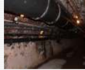
Kanalisation in Paris
